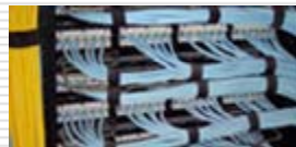
Low Voltage Systems
