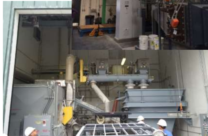
West Boise WWTF, Boise, ID
