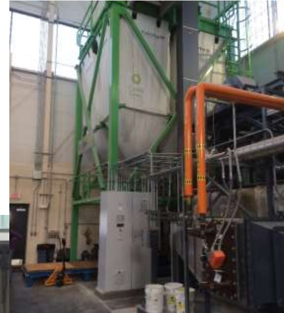
Nine Springs WWTP, Madison, WI
