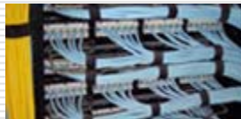
Low Voltage Systems
